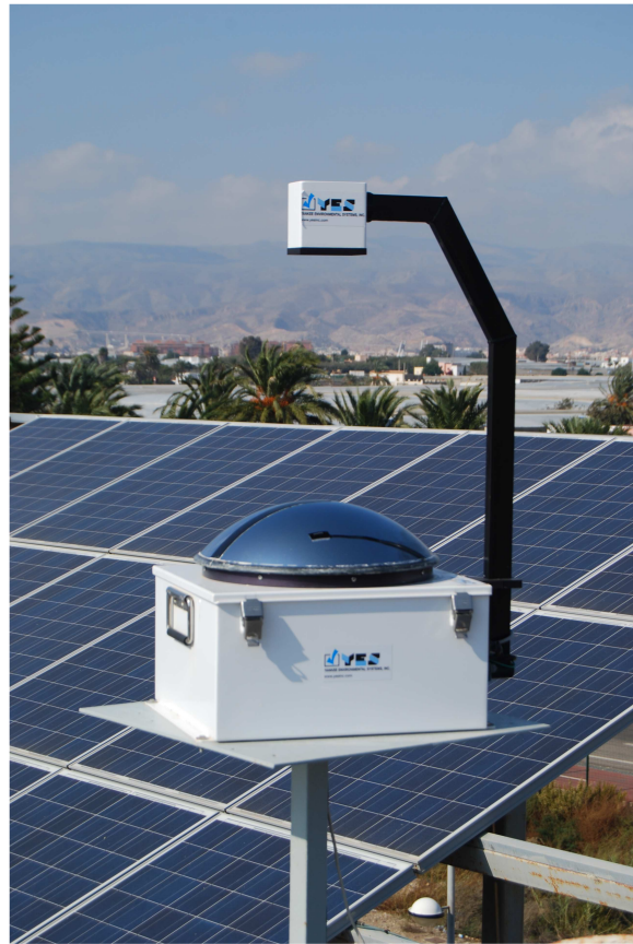
Figure 6. TSI-880 installed in CIESOL.
