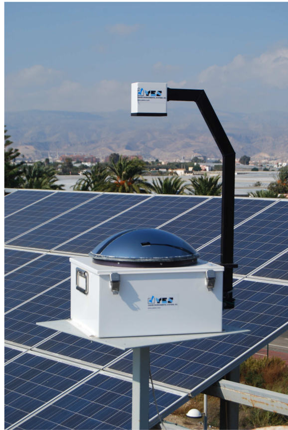
Figure 6. TSI-880 installed in CIESOL.
