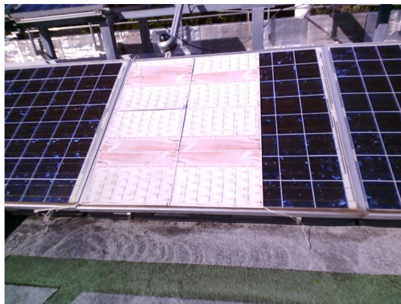
Figure 3. Experimental PV plant with partial shading.
