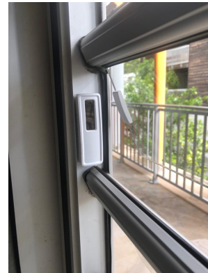
FIGURE 3. Opened window (called louvers) with magnetic contact
