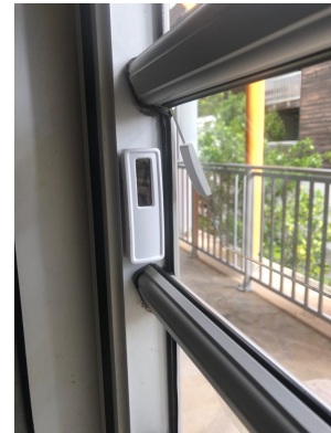
FIGURE 3. Opened window (called louvers) with magnetic contact
