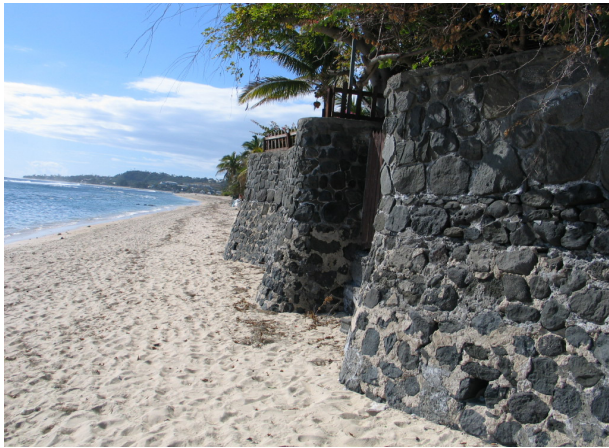
Fig. 5. Sustaining wall of a private property encroaching on L'Ermitage beach
